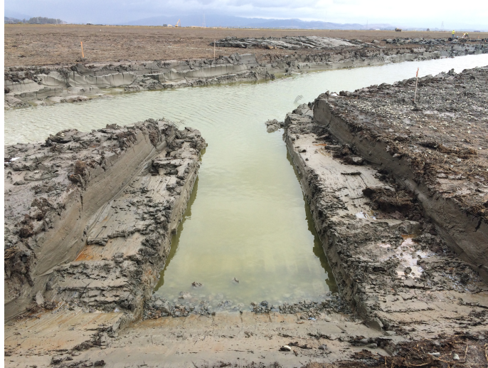
Figure 12. Seven lateral starter channels were cut into the main channel alignment. With the constant flow of water in and out of these starter channels, longer, meandering natural channels are expected to form over time.
