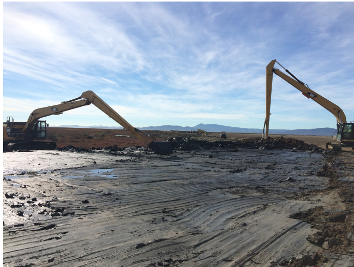
Figure 13. Because construction on the main channel alignment and other projects aspects was complete by 11/15/2015, Hanford was able to complete the formation of the transition ramp in the remaining two weeks of our construction permit window. The final result is approximately 9 acres of transition ramp 120ft wide and 3ft tall from marsh plane to levee, a (40:1) slope, gently sloping habitat ramp. This portion of the project was projected to be shaped in 2017 and
